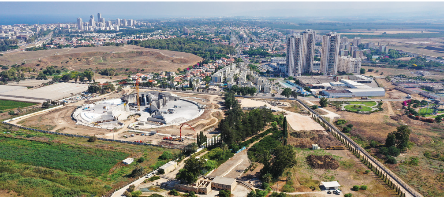
Construction of the Shrine of ‘Abdu’l-Bahá continues to advance following the fire caused by an accident in April. The cleaning is set to be completed in the coming days. Photo: Bahá’í World News Service
